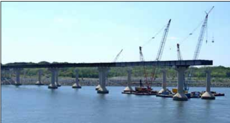
Above - Ron Stubblefield got this shot of the new P&L bridge across the Tenn. River next to the future hwy 62 bridge.
